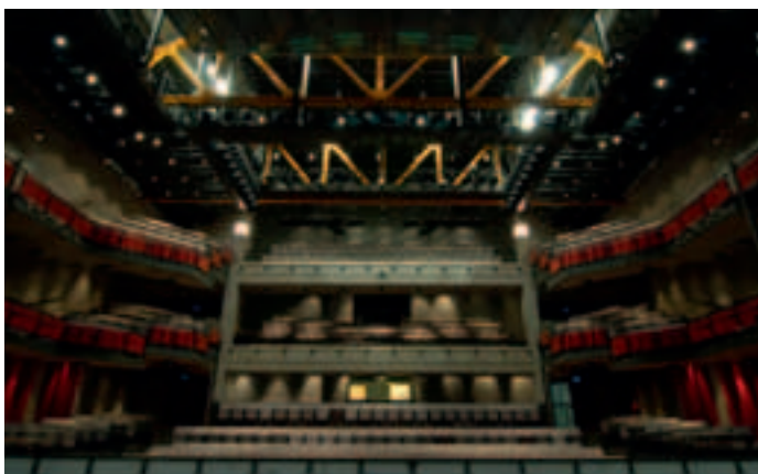
All lights burning, all dimmers functioning
